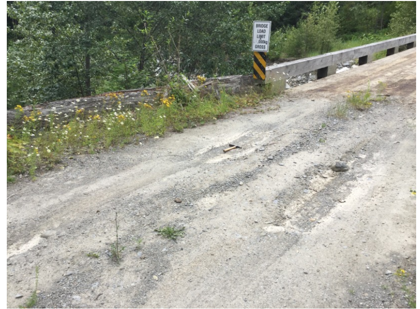
Typical Potholes in Approach & Rotten Guide Log
