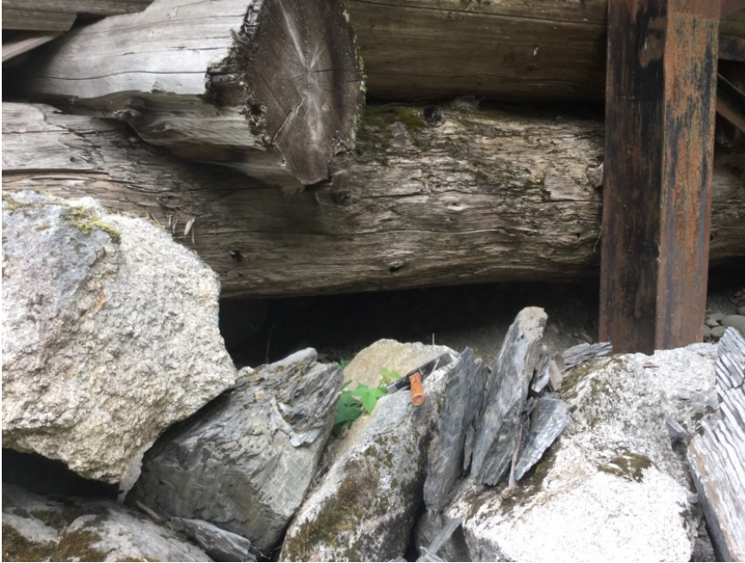
Left Abutment Upstream Corner Scour
