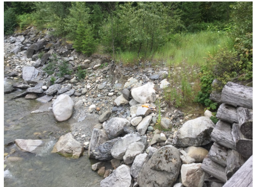
Left Bank Erosion at Upstream Corner
