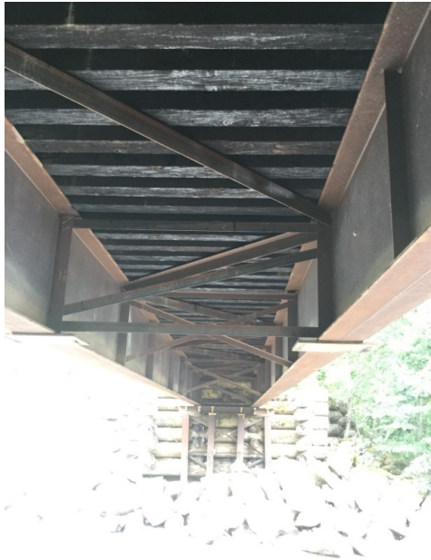
Girder Condition & Removed Pier Bearing Plates
